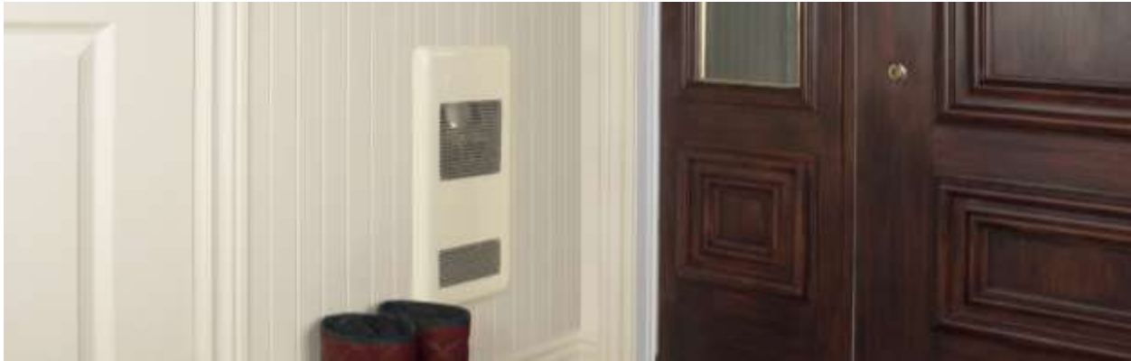
Figure 2 - Electric resistance wall heater
